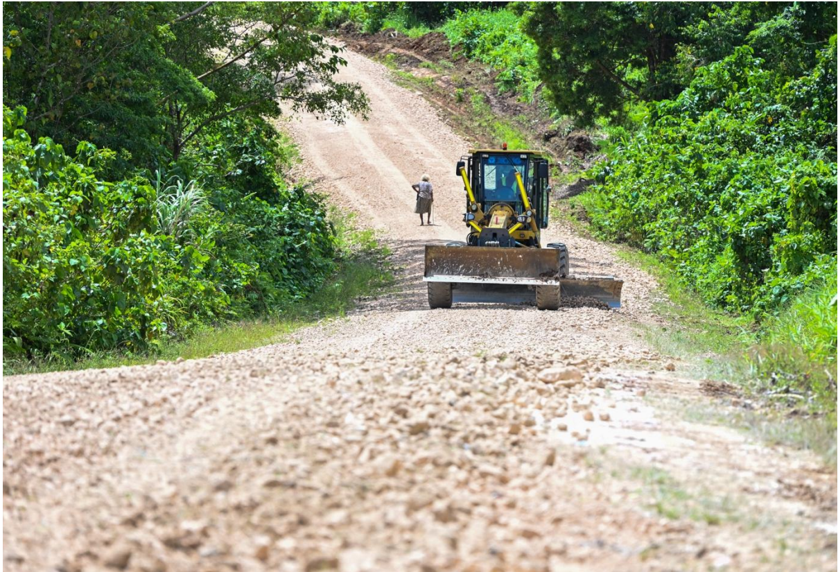
Photo 4 – The road works have re-opened access to key agricultural areas in Malaita.
